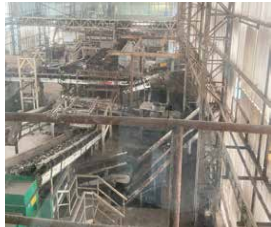
Figure 17: Waste Segregation at the Waste-to-Energy Plant
